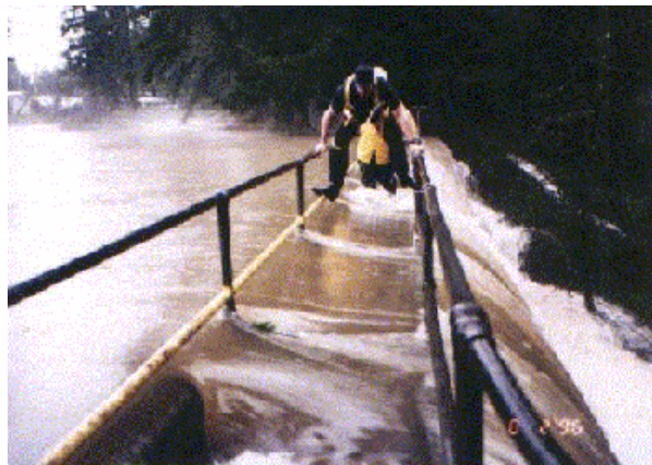
Figure 2. Flooded Dam, Lacamas Lake Dam, Camas, WA, 1996
